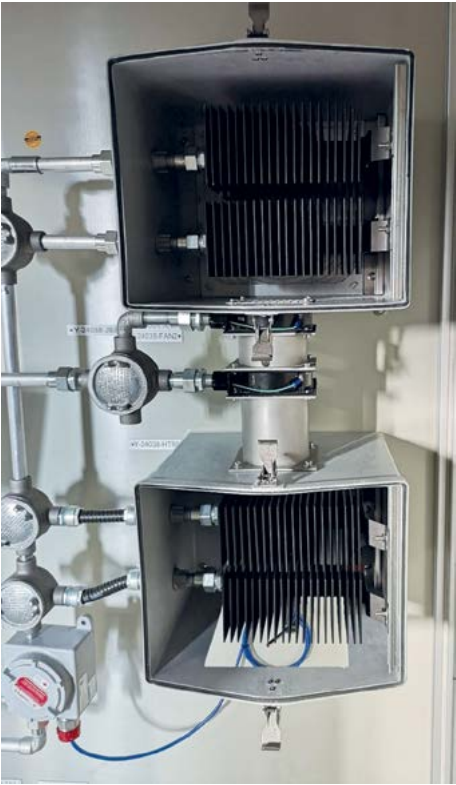
Redundant ventilation fans with pre-warming system.
