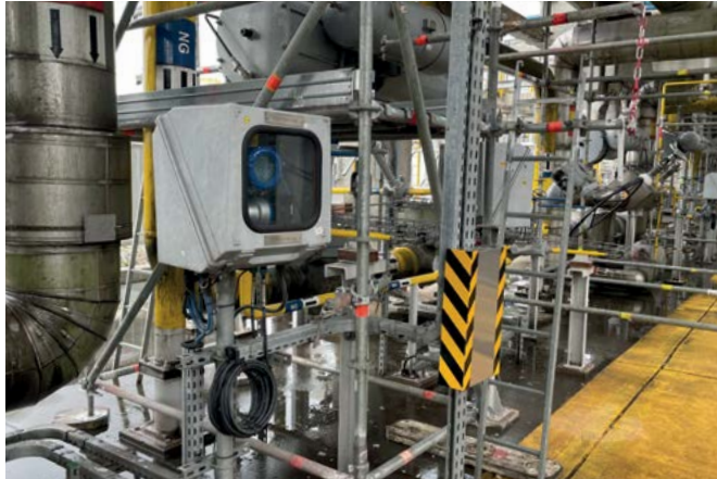
Temperature controlled transmitter enclosure for LNG terminal.
