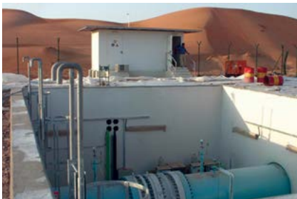
Advanced insulation is a key aspect of these shelters for the instrumentation/SCADA stations on a Middle East water pipeline, allowing totally passive cooling to limit the extremes of day and night temperatures.
