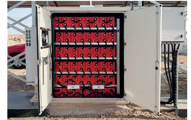
Cooled battery shelter.
