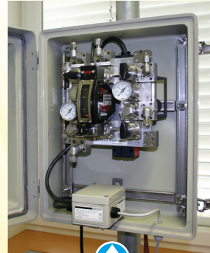
↑ INTERTEC produces several application-specific heaters such as this conduction heater for SP76 instrumentation substrates (mounted behind substrate).
